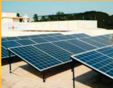
Solar 7.5 KVA Panel & Stand Solar Power Plant
