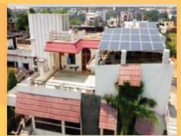
Solar 5 KVA Panel & Stand Solar Power Plant
