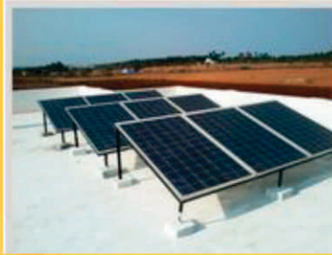
Solar 3 KVA Panel & Stand Solar Power Plant
