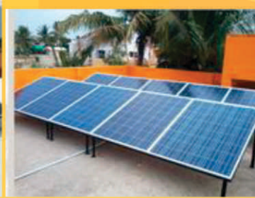
Solar 3 KVA Panel & Stand Solar Power Plant
