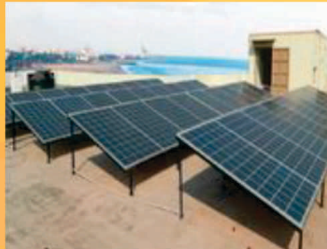
Solar 10 KVA Panel & Stand Solar Power Plant
