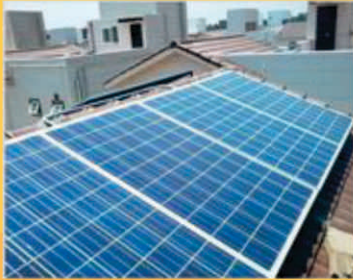
Solar 1 KVA Panel & Stand Solar Power Plant
