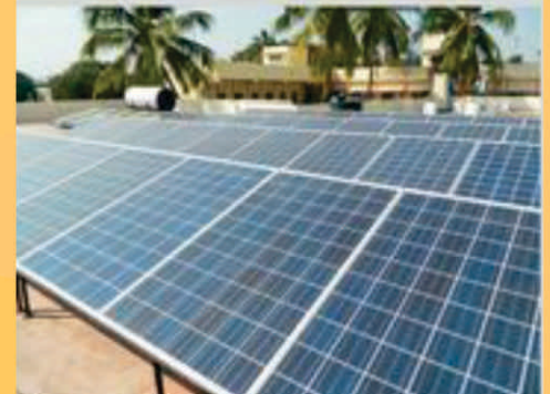
Solar 25 KVA Panel & Stand Solar Power Plant
